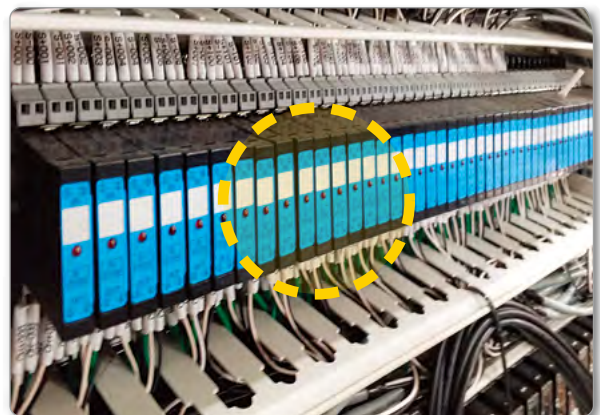
Water Treatment Control Panel
